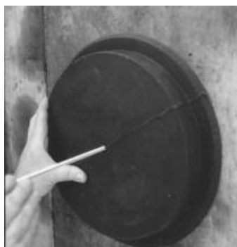
After nailing end cap to form, drive (threaded rod*) through the end plate and form and (thread nut*) on other side. Note: Remember to measure the (threaded rod*) to match the length of the sleeve.
